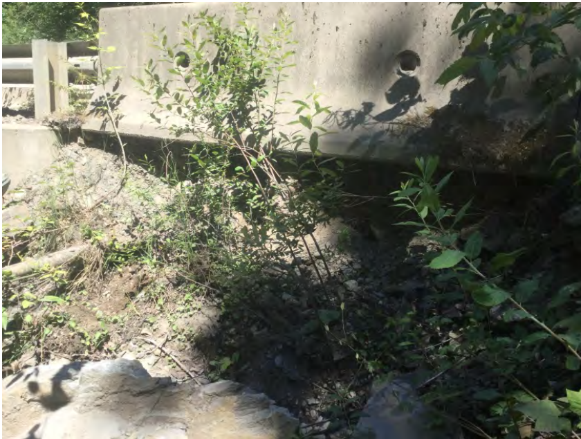
Fill under no post barriers on down stream left bank failing
